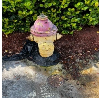
Fire hydrant needs to be replaced
