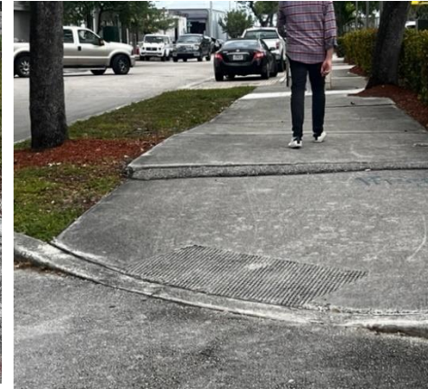
Sidewalks are uneven
