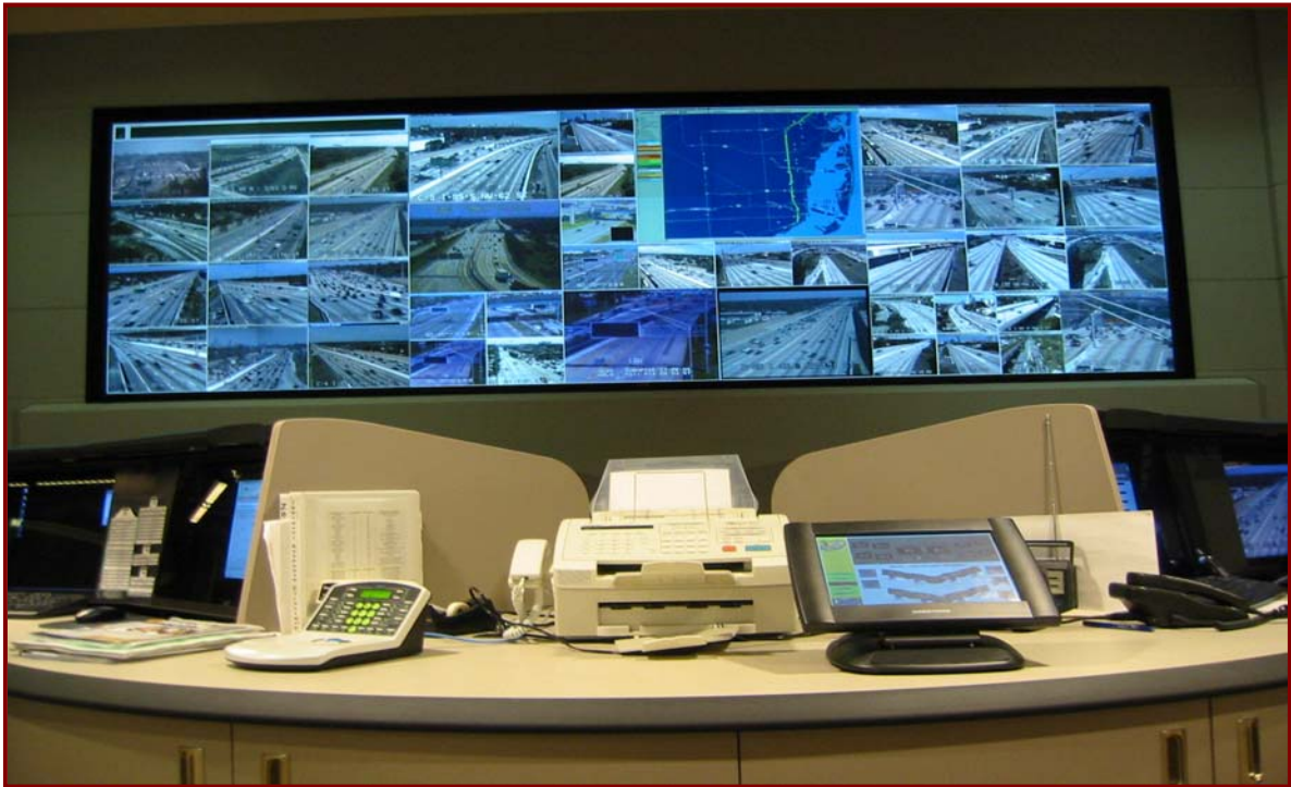
Traffic Management Center Monitoring Screens
