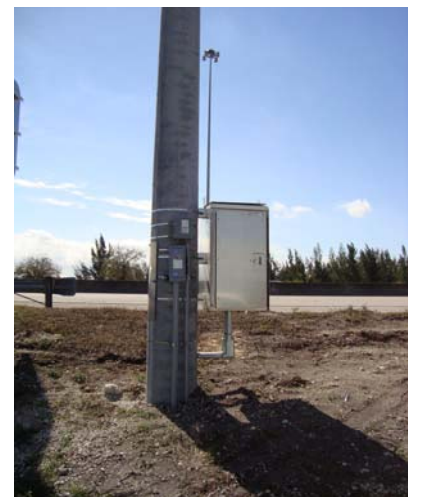
ITS Surveillance equipment
