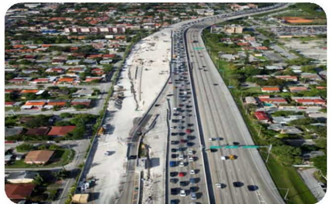
SR 836 at former Wing Gantry Location looking west
