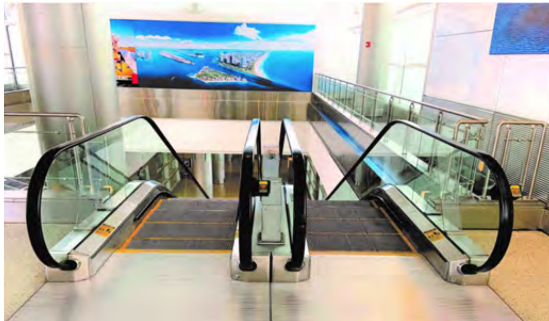
Escalators at MIA
