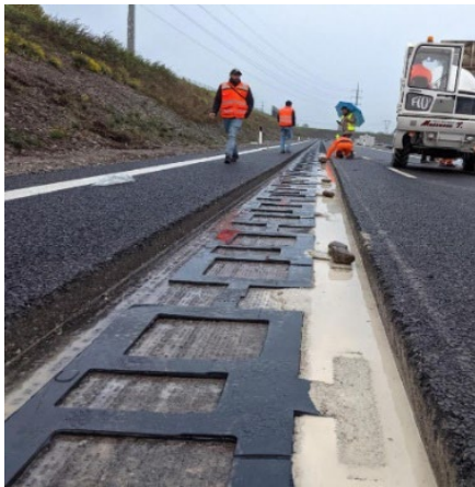
Figure 6-10 Dynamic Wireless Charging
